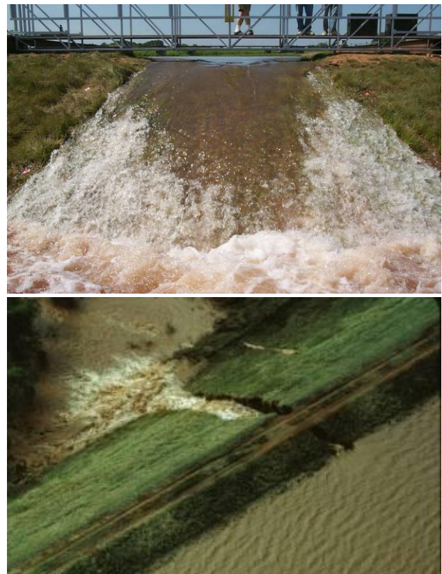
Figure 1. Overtopping and internal erosion of dams
