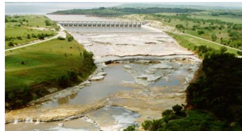
Figure 8. Eroded auxiliary spillway.
