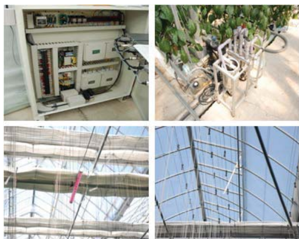
Figure 10. Greenhouse Facilities and Power Controller
